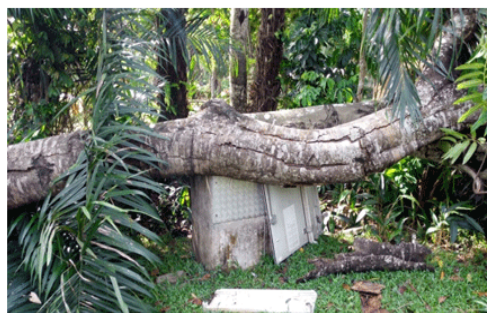
Plate 2: Tree fall with impact on telecom panel
